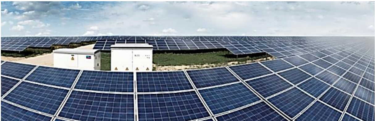
Figure 4 Example of typical Power Conversion Units
